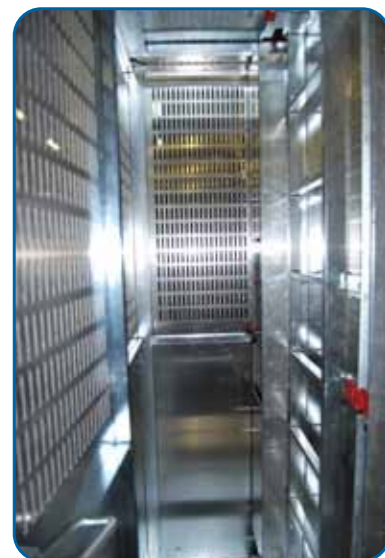
Interior de cabina Interior of the cabin
