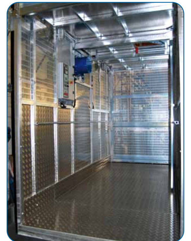
Interior de cabina de T1 Cabin interior in T1
